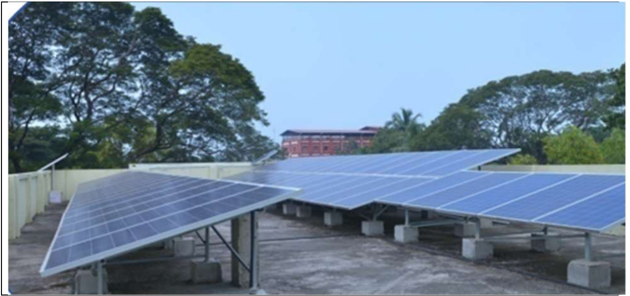
Solar panel units
