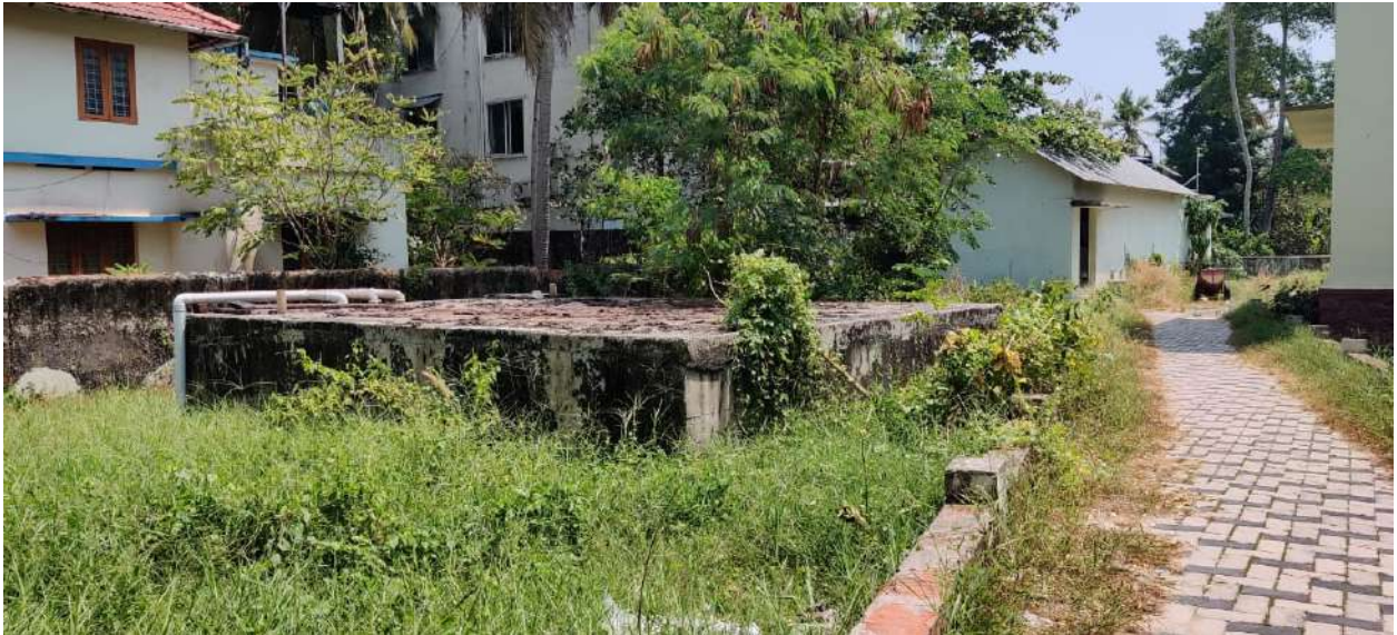
Ground water recharge unit
